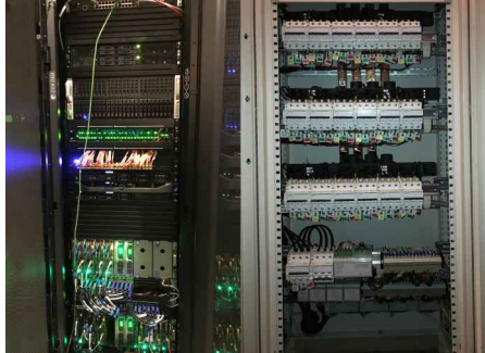
Data Center monitoring
